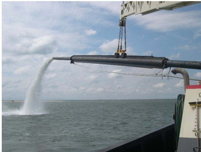
A shipboard view of the sidecast dredge, the Fry , in action last summer along the Bogue Inlet connecting channel.
